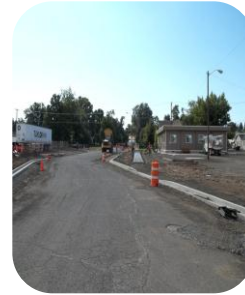
South Mill Street under construction at the time of press shown above. This project will be complete by the end of September.
